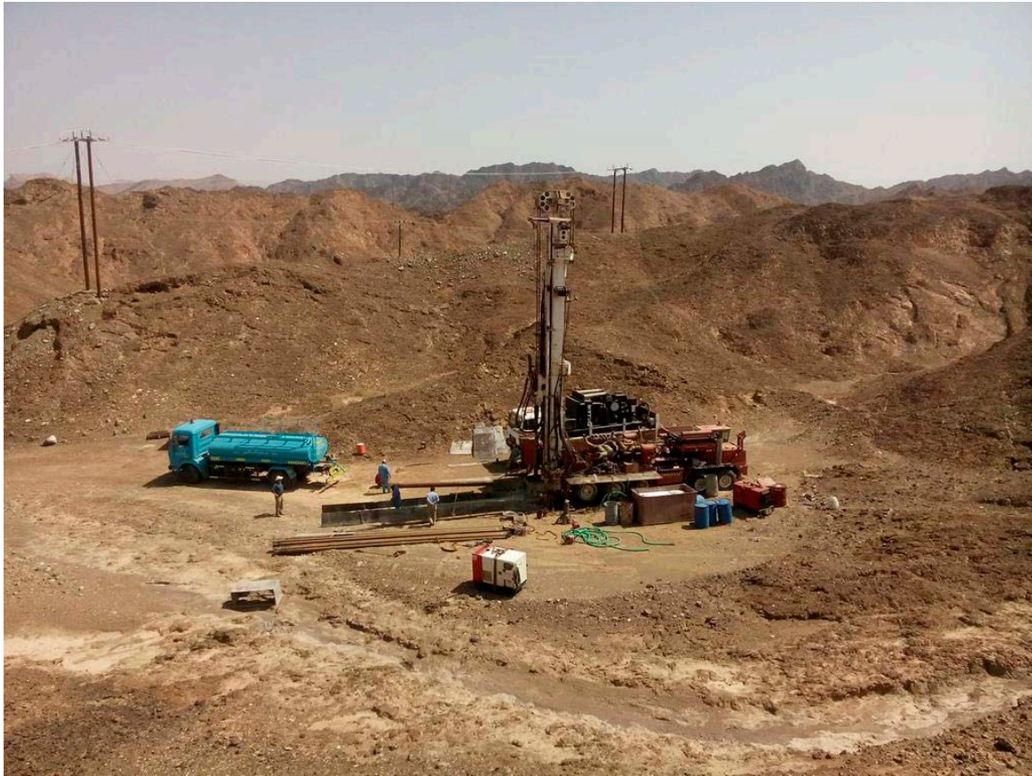
Figure F1. Photograph of Site BA2 during rotary drilling operations, looking southwest. Image credit: Nicolas Bompard.
