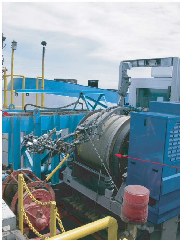
Old heave compensating system
