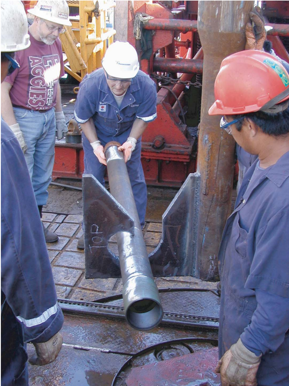
Figure F8. Fishing tool fabricated to retrieve the failed 4½ inch casing from inside the reentry cone and casing of Hole U1301B.
