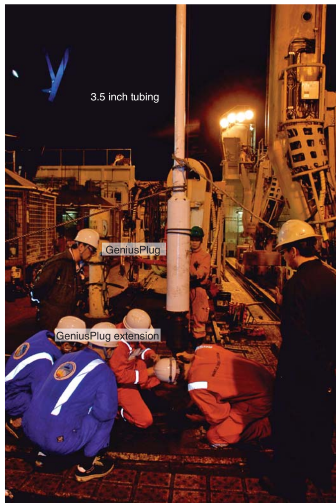
Figure F5. GeniusPlug (white paint) and tubing joints on rig floor before deployment during Expedition 332.
