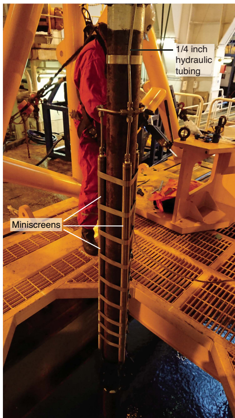
Figure F4. 3.5 inch tubing bullnose at the bottom of the LTBMS assembly, with position and orientation of pressure port (P1) miniscreens.
